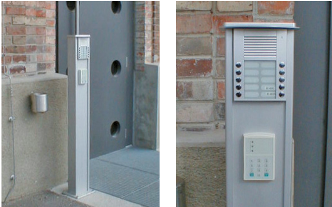
GAS 160 - Vienna Fairground access control
