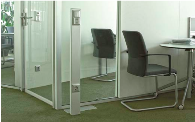
GAS 100 - Office building Borealis Innovation Headquarters Linz
