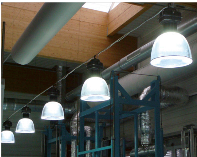
EDP No. 108559, Hall lighting plastics industry
