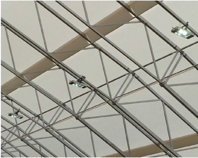
EDP No. 91079, Hall lighting
